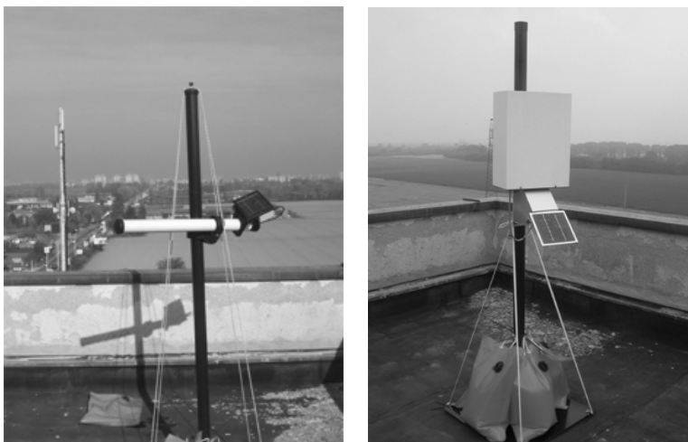
Figure 2. Examples of mounted monitoring station
